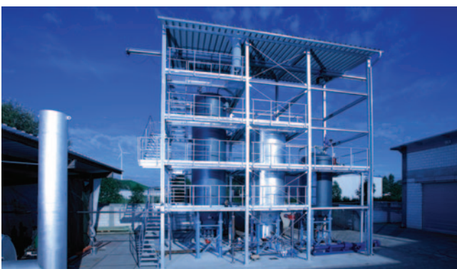
AVAC02's demo plant for hydrothermal carbonisation
